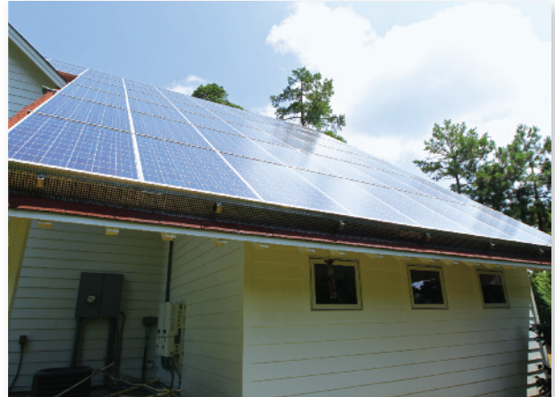
View of the Staffords' solar panels from the ground.
